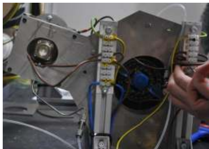
Figure 55 - Electrical Interface for the test rig
